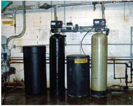
An industrial water treatment system
