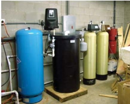
Lake water treatment here includes disinfection and filtration
