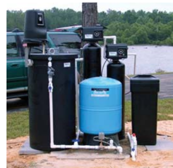
A system with a combination of disinfection, iron/manganese filtration and water conditioning
