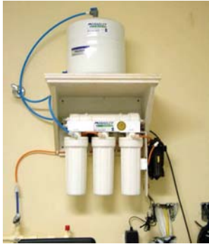
An RO purification unit
